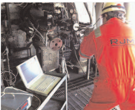
Figure 2. Inserting the anemometer into the furnace via the oil burner carrier tube. The position of each burner is entered into the software along with the position of the measurement point
